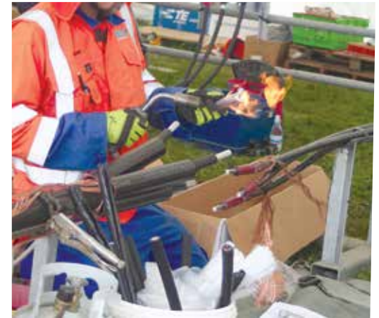
HT CABLE JOINTER
